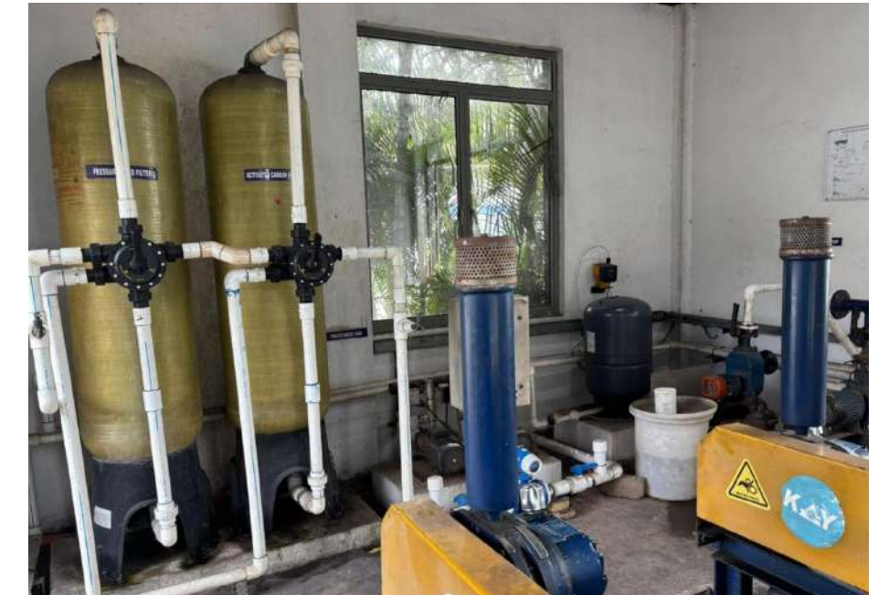
STP: Sewage Treatment Plant
